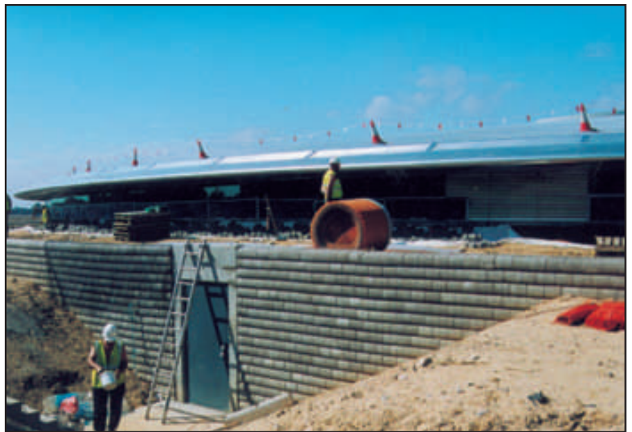
Porcupine blocks form the vertical face of the wall at a low level access door into the treatment plant
